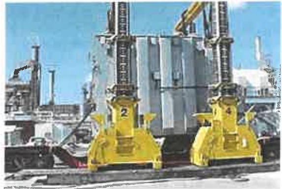
Power System Expansion Convent, LA
